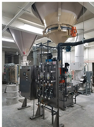
The new lime slaker at the Ottawa Water Treatment Plant. (photo submitted)
